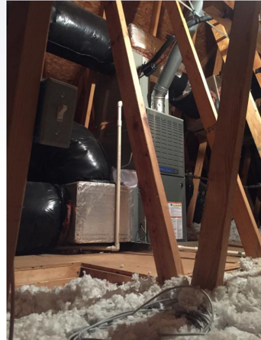
Gas furnace in attic
